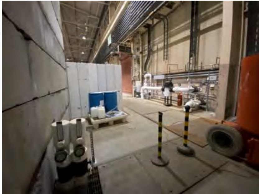
Figure 6: View of the HVAC Pipes
