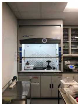
Figure 2. Upgraded/New fume hood with automatic sash
