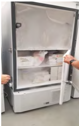
Figure 3: Inside of a new freezer from the “Freezer Farm”
