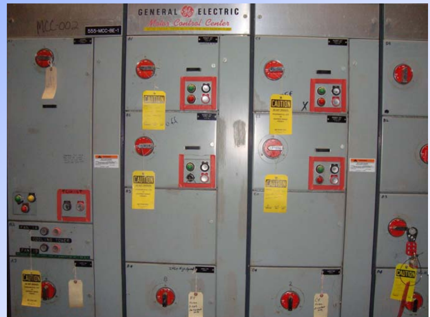
480V Motor Control Center
