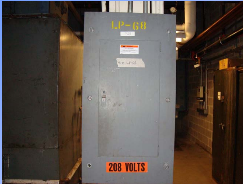
208V Lighting Panel
