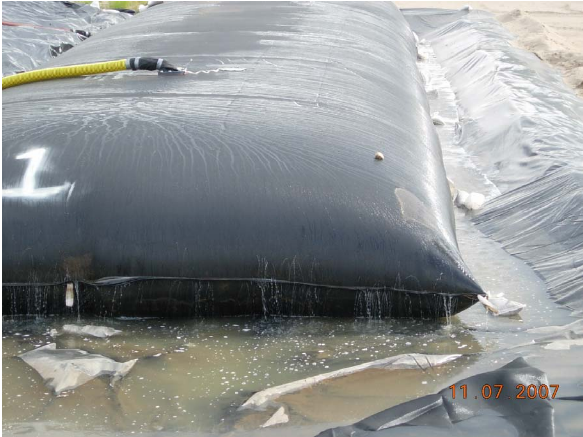
Figure1. Water being extracted from the biosolids
