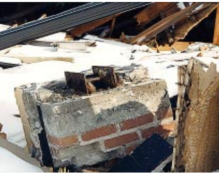
Cemented to a wall pillar is one of the metal brackets that attached a roof truss to the wall via a stub column, but that concealed the condition of the end of the stub column. — Photos by Peter Horton
