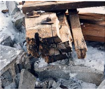
One of the two stub columns on Bldg. 424's western wall that had deteriorated by dry rot due to water infiltration.
