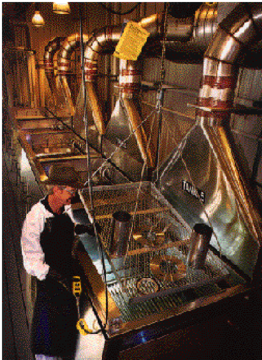
Helper Jeff Raynor at the CSD's new Central Degreasing Facility.
