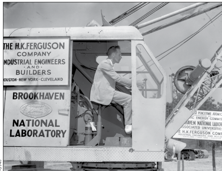
At the controls of a crane belonging to H.K. Ferguson Company, the contractor that built the Brookhaven Graphite Research Reactor (BGRR), BNL project leader Lyle Borst ceremoniously scooped out a bucketful of earth at the groundbreaking ceremony on 11 August, 1947.
