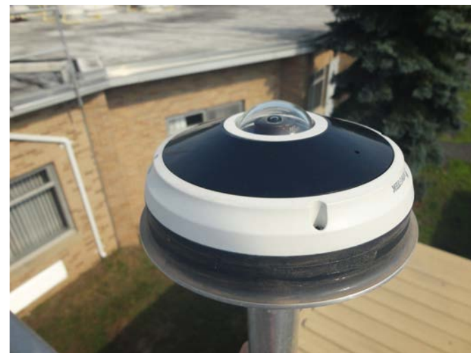
HD Sky Imager mounted on BNL Bldg 490 roof
