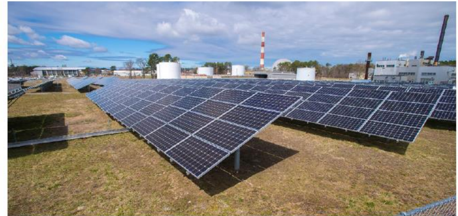
View of the Northeast Solar Energy Research Center (NSERC)
