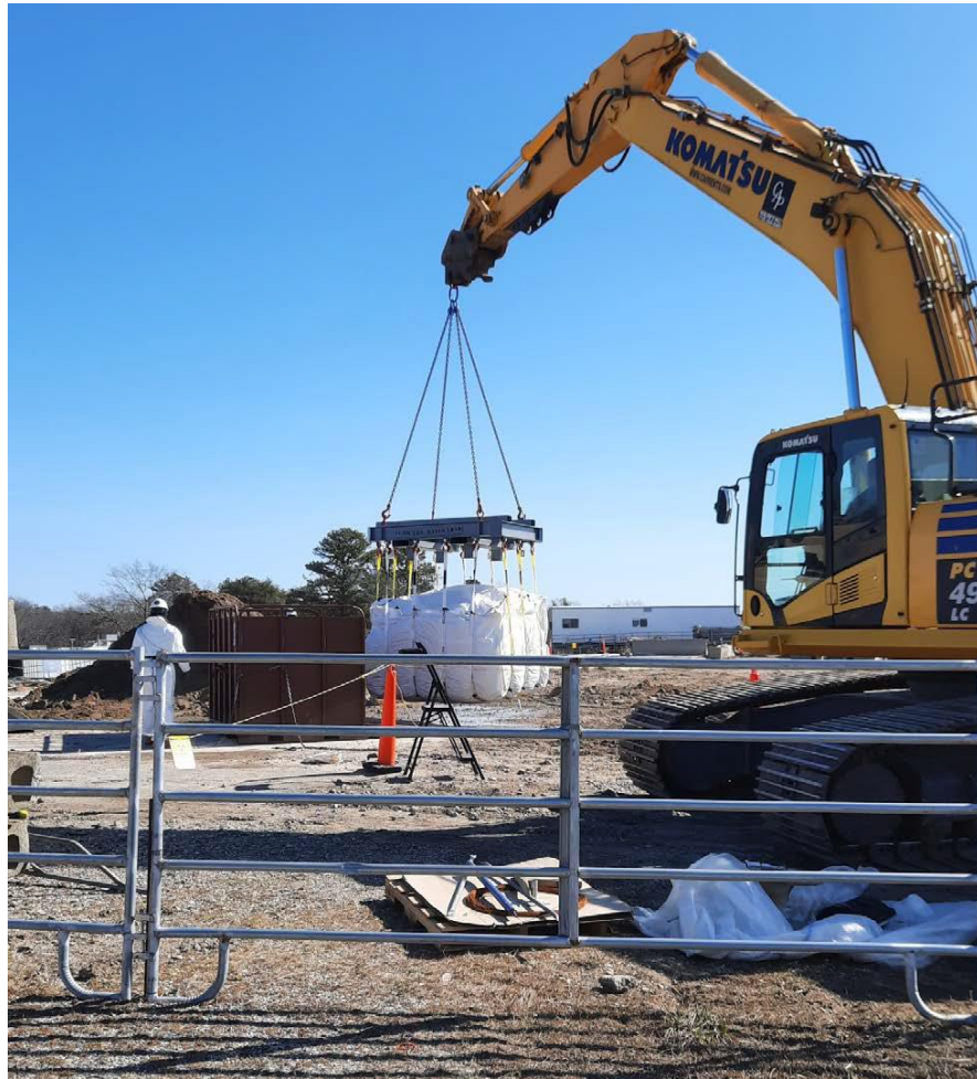
Loaded and screened 10 cubic yard supersack being removed and staged for transport to the railyard
