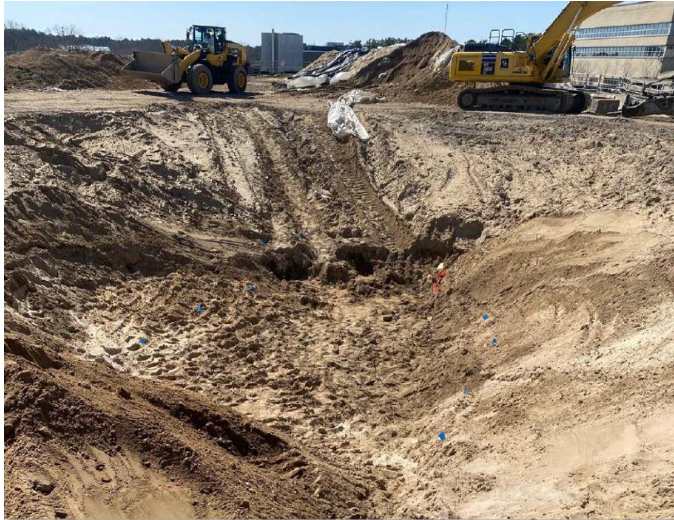
View of silencer excavation looking east. Silencer footprint is within the blue flags.
