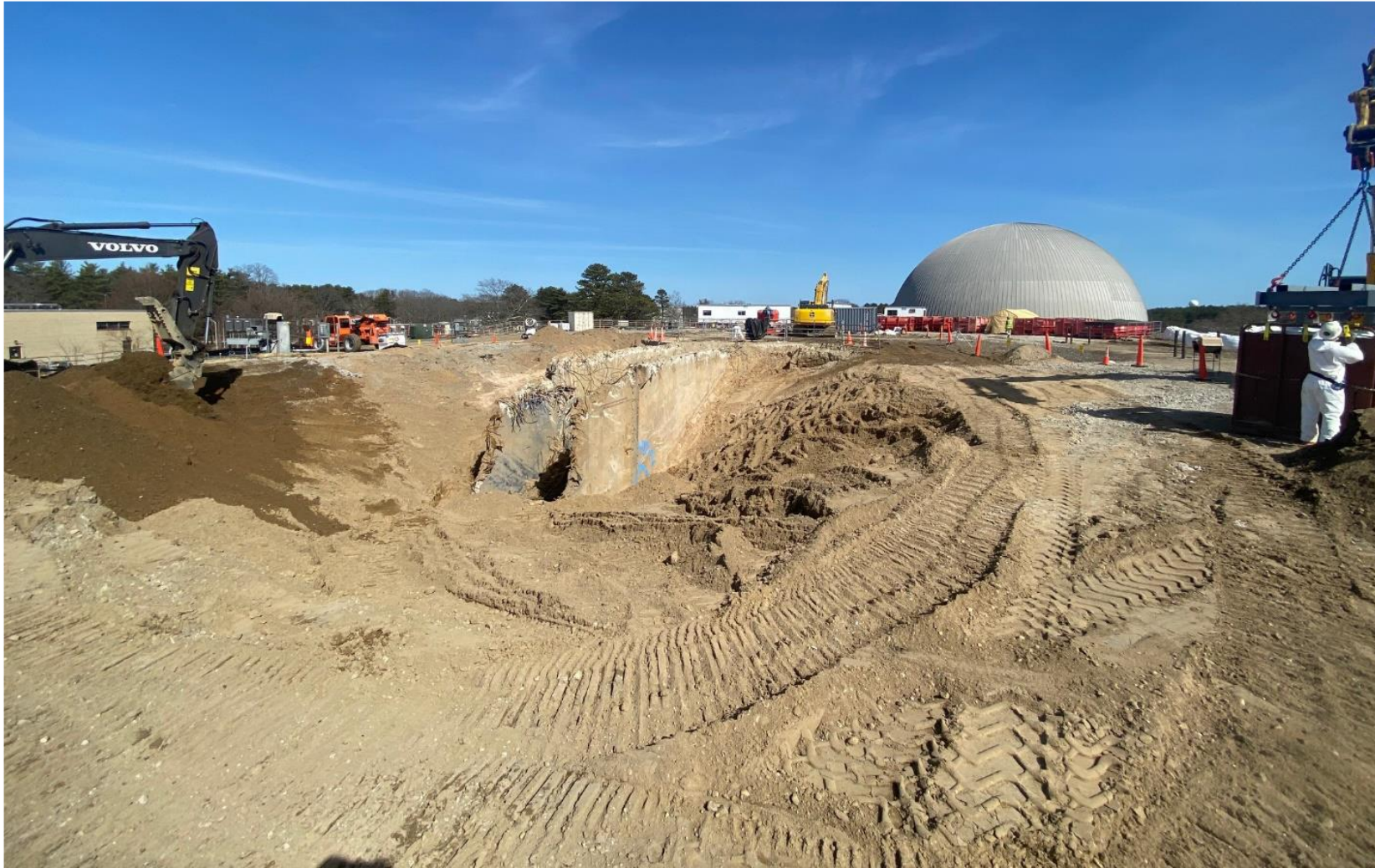
View looking east of the exposed silencer and grading of surrounding soil to allow for demolition
