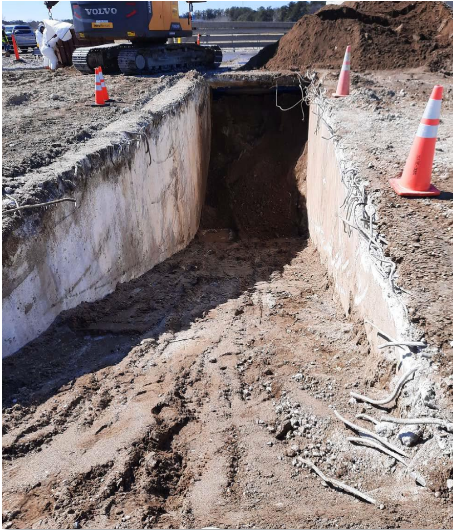
View of the exposed silencer looking west
