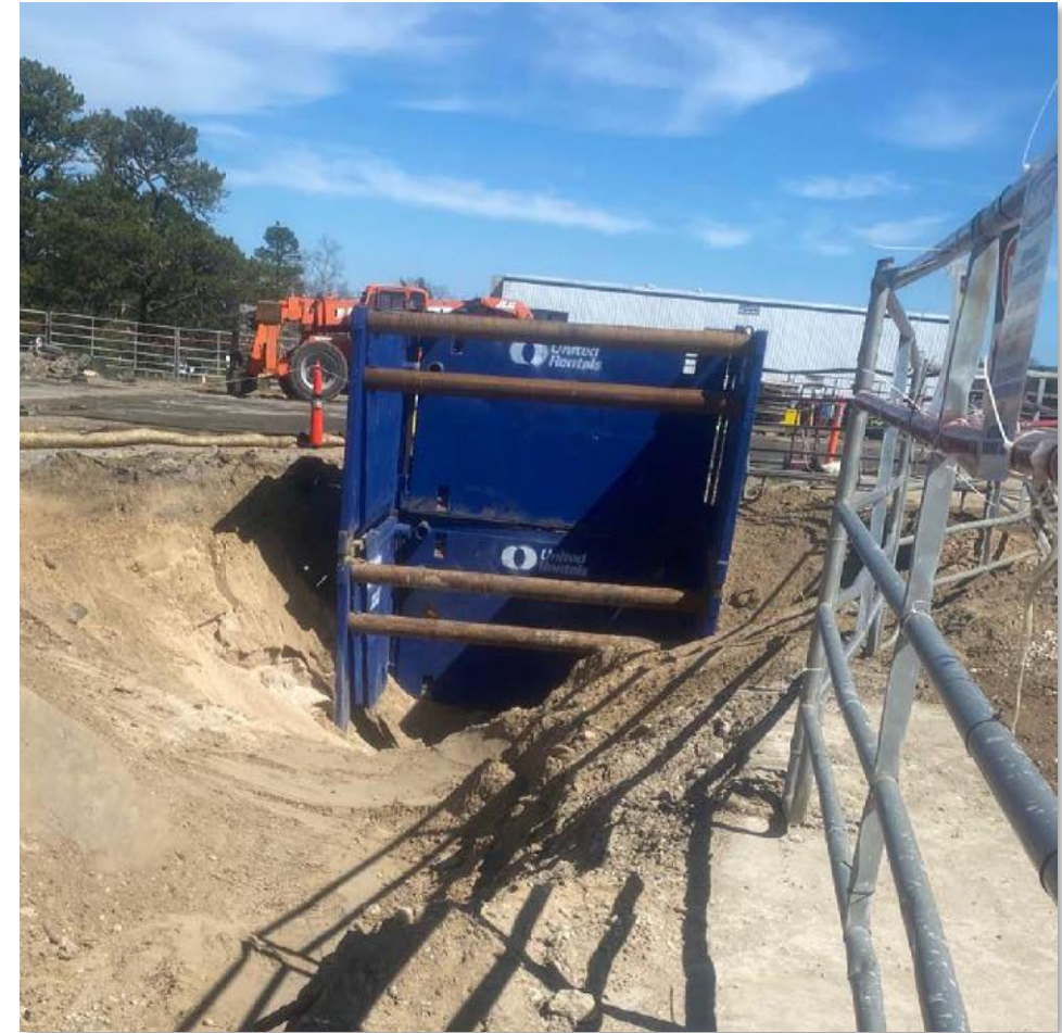
View looking east at the installed shoring box in the stack drain tank excavation
