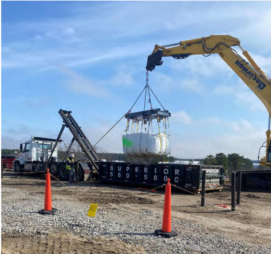
10 cubic yard soil supersack being weighed and loaded for transport to the rail yard
