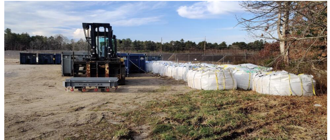
Intermodal containers and soil sack staging area at the railyard in preparation for transport
