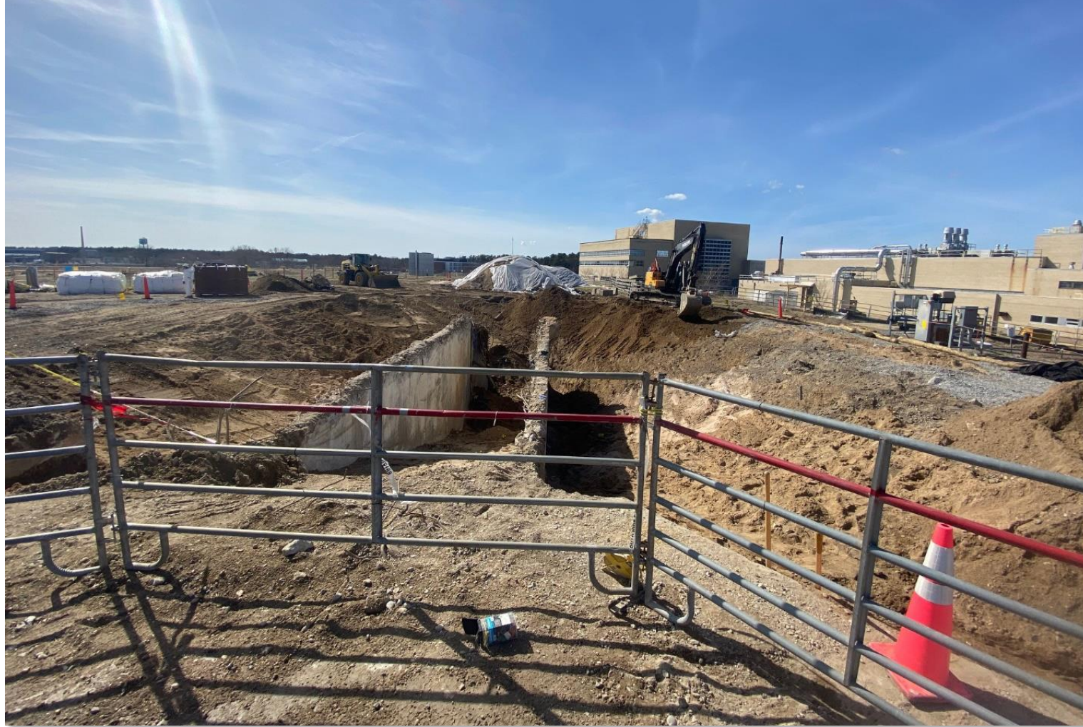
View of the exposed silencer looking west from the pedestal
