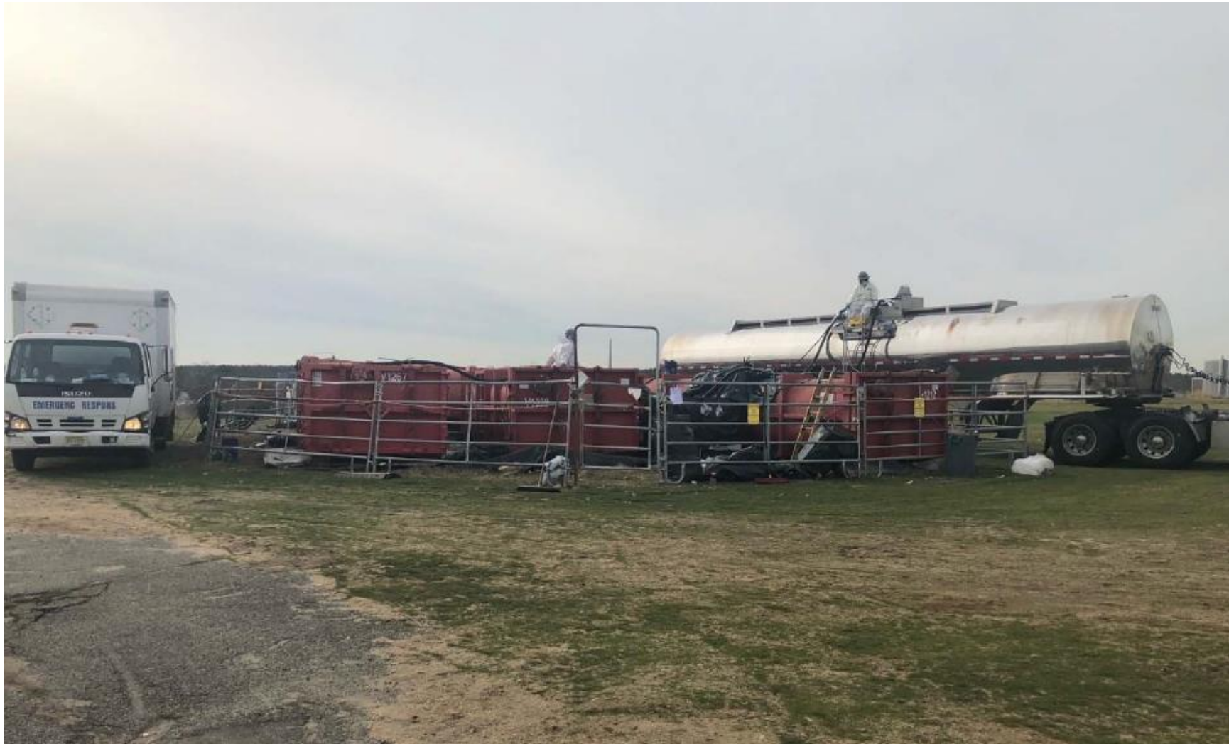
Wastewater from paint abatement project being transferred from temporary storage tanks to tanker trucks for disposal (DEC21).
