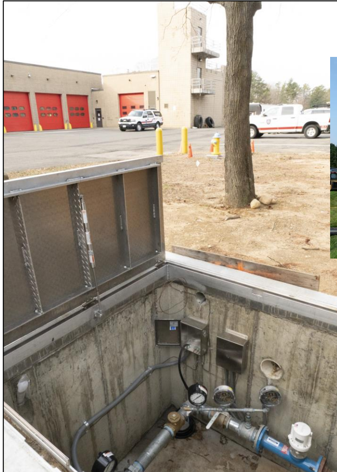
Extraction Well Vault at Current Firehouse
