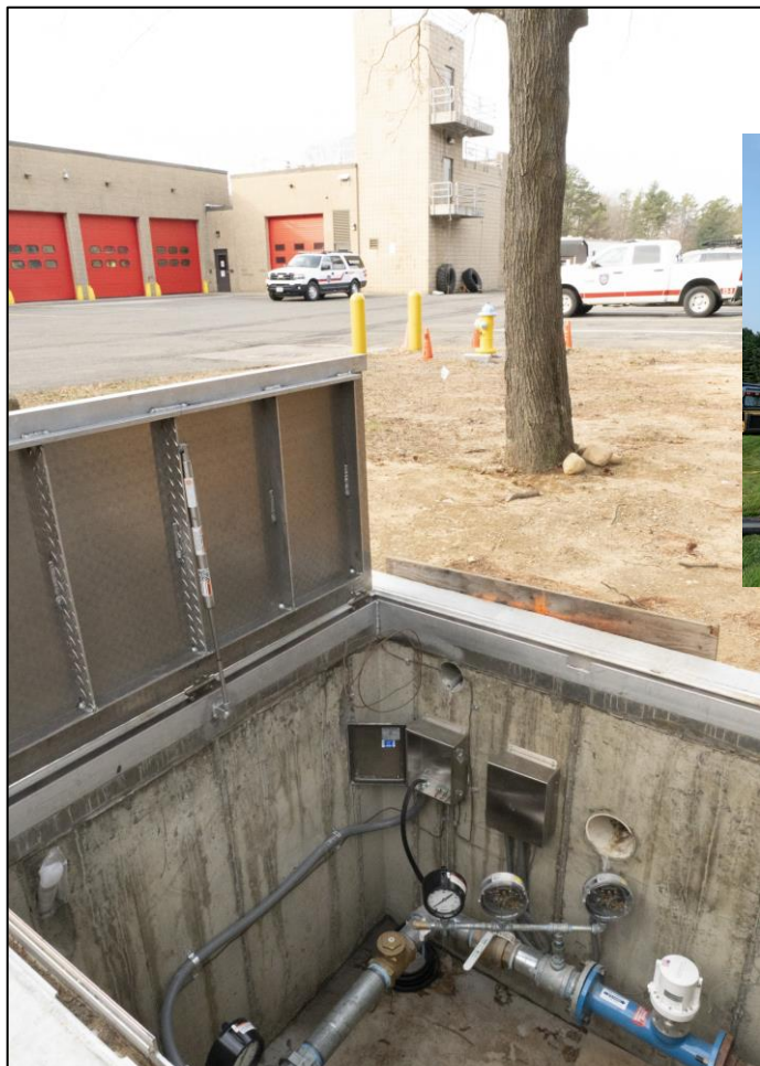
Extraction Well Vault at Current Firehouse
