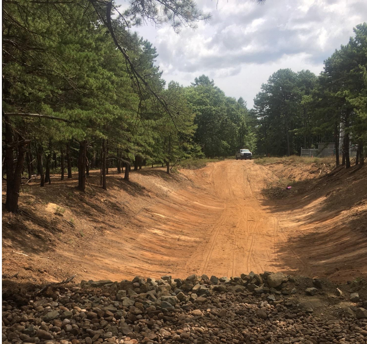
Recharge basin for the Current Firehouse/Building 170 Treatment System
