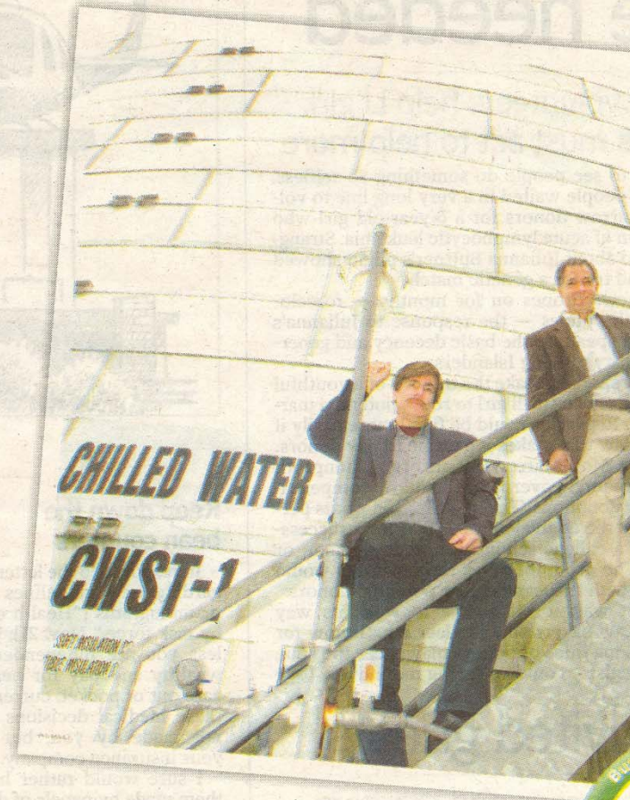
Mark Toscano (left) and Peter Pohlot climb the stairs of Brookhaven National Laboratory's 71-foot chilled water facility, which has reduced electric demand by 2,000 kilowatts during peak daytime periods, saving over $2 million in energy costs since 1998.
