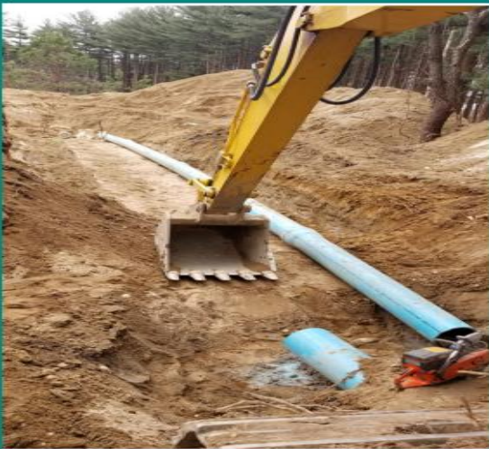
Photo: Installation of underground piping connecting groundwater extraction wells to a PFAS treatment system at BNL.
