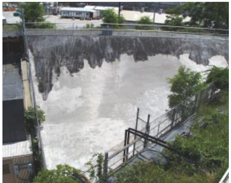
Figure 2-16. Guniting Cap Installed Over g-2 Area Prevents Rainwater from Reaching the Activated Soils and Potentially Contaminating the Groundwater.
