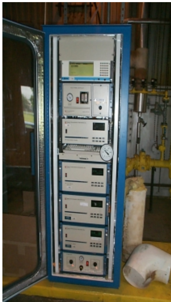
Figure 4-6. Central Steam Facility Continuous Emission Monitoring Analyzers.
