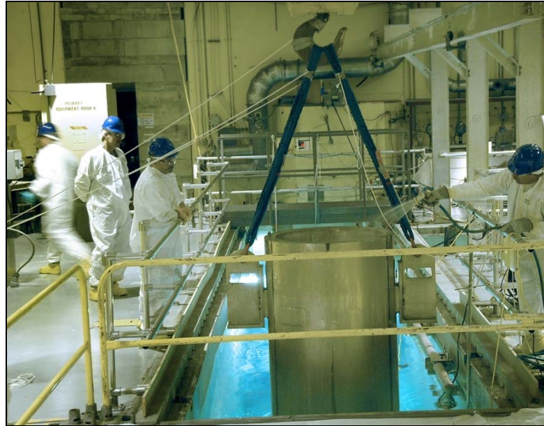
Figure 3-10. Shipping cask being lowered into the fuel pool.
