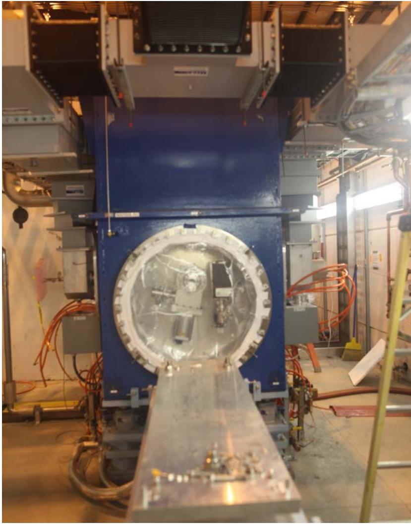
Figure 6. The cryomodule of the SRF gun seen from the cathode insertion port side.
