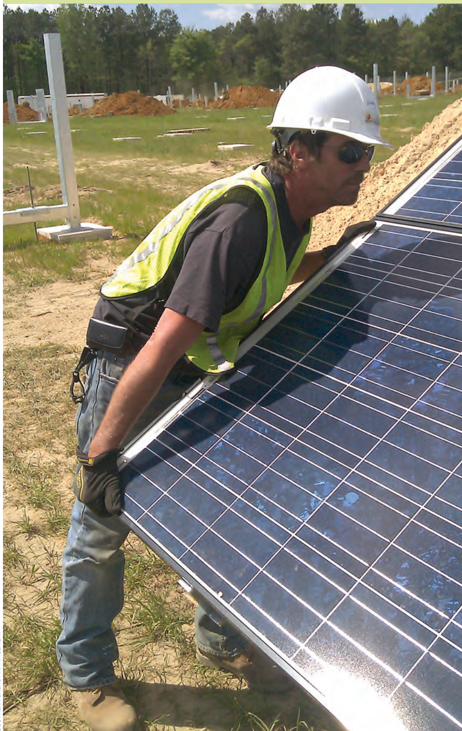
SOUTHERN ENERGY MANAGEMENT
