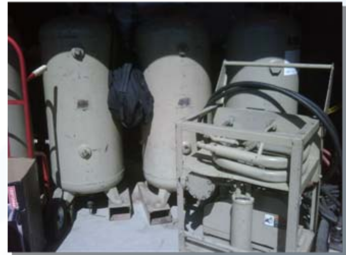
R-11 refrigerant recovery equipment
